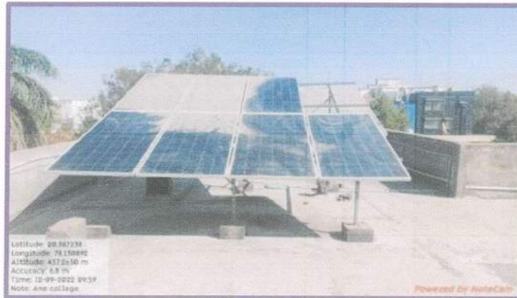
Photograph of Roof Top Solar PV Plant:
