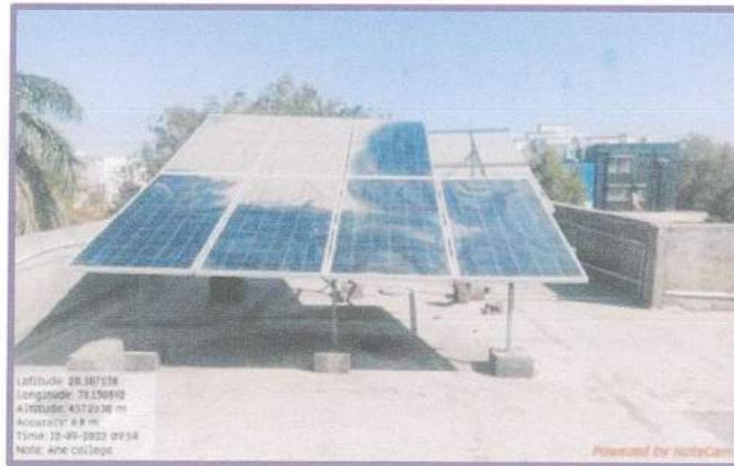
Photograph of Roof Top Solar PV Plant:
